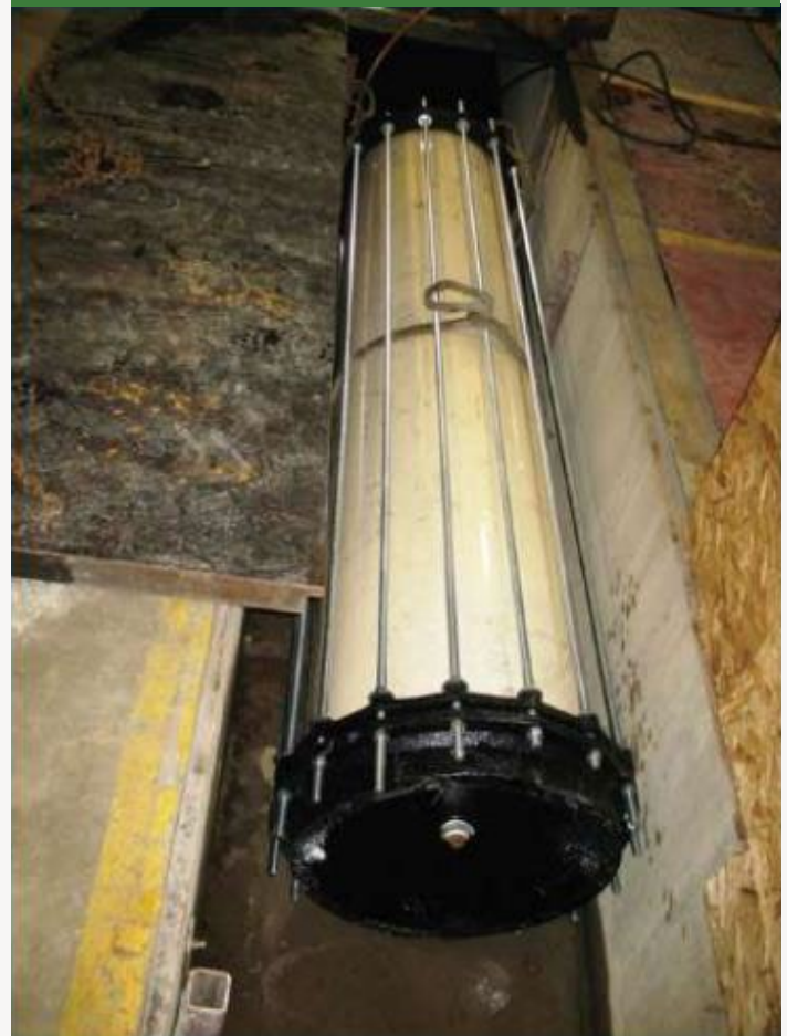
FIGURE 1: 20-YEAR-OLD PVC FORCE MAIN THAT MET AWWA STANDARDS FOR NEW PIPE
